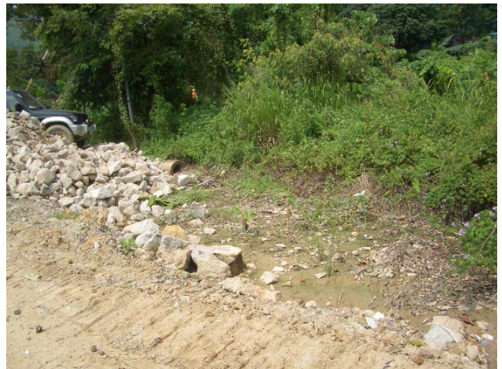
Stagnant water was cleared at MUP01.
