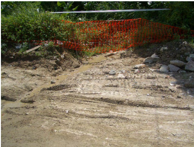
1. Sludge observed at TKL02. The contractor is advised to implement certain mitigation measures such as installing desilting facilities
