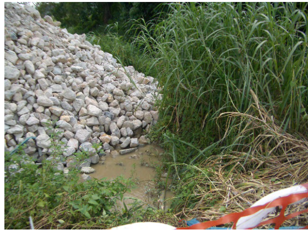
2. Muddy water observed at TKL07. The contractor is reminded to prevent any direct discharge of muddy water
