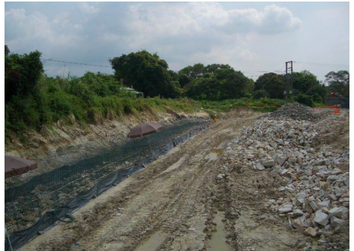
Stagnant water was cleared at TKL07.
