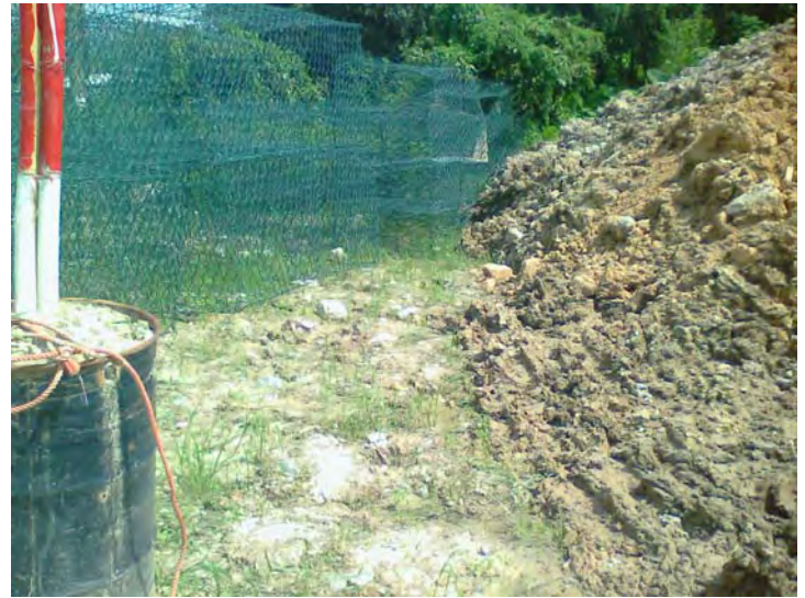
Stagnant water was cleared at TKL07.
