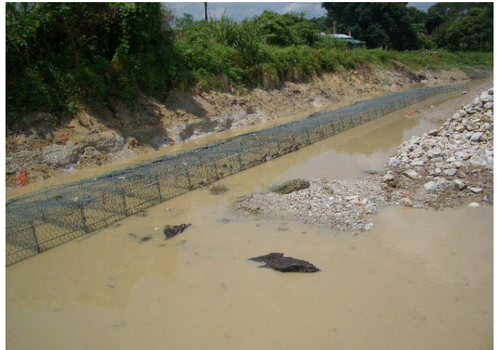
2. Stagnant water observed at TKL07 . The contractor is reminded to prevent any accumulation of stagnant water
