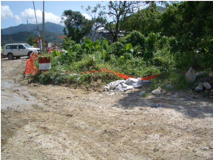
Filter was set up at TKL07.
