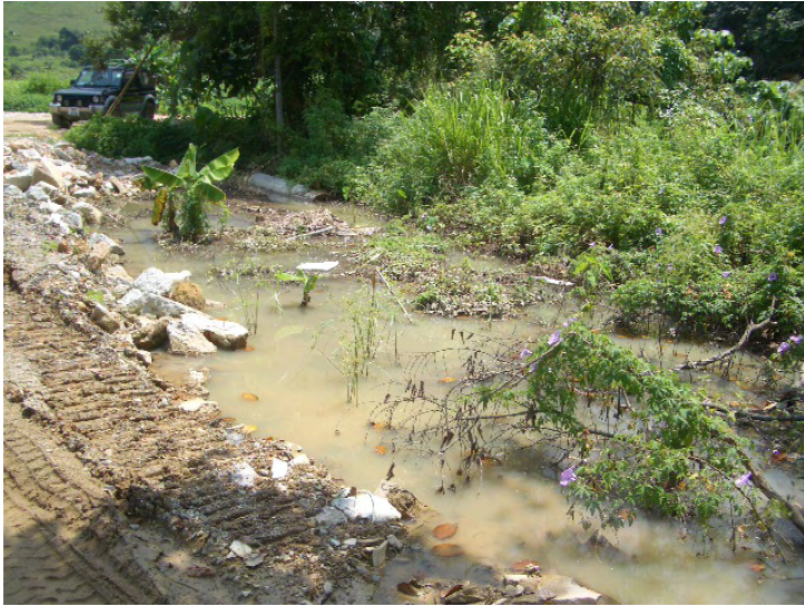
3. Stagnant water is observed at MUP01. The contractor is reminded to remove any stagnant water on site to eliminate mosquito breeding.
