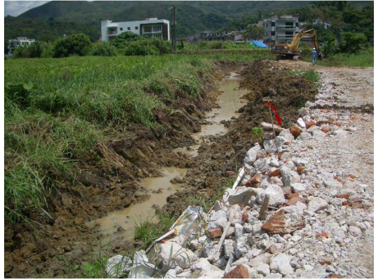
4. Muddy water is observed at MUP01. The contractor is reminded to implement relative mitigation measures, such as placing sand bags, and desilting facilities before discharge
