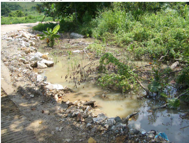
3. Stagnant water is observed at MUP01. The contractor is reminded to remove any stagnant water on site to eliminate mosquito breeding.
