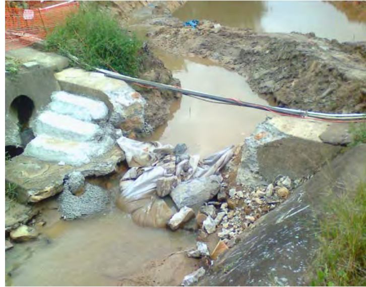
Filter had been set up for desilting purpose.
