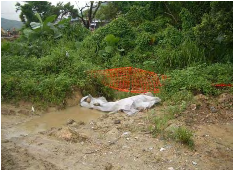
Damaged filter has been rectified at TKL07.
