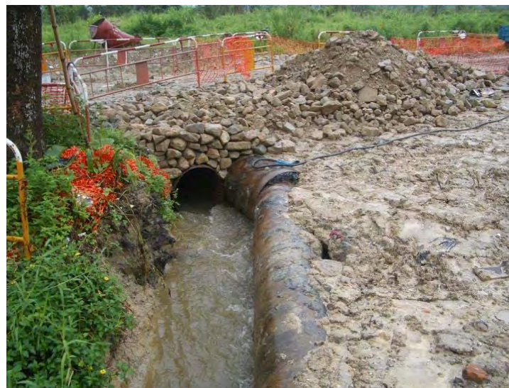
Damaged earthbound has been rectified at TKL07.
