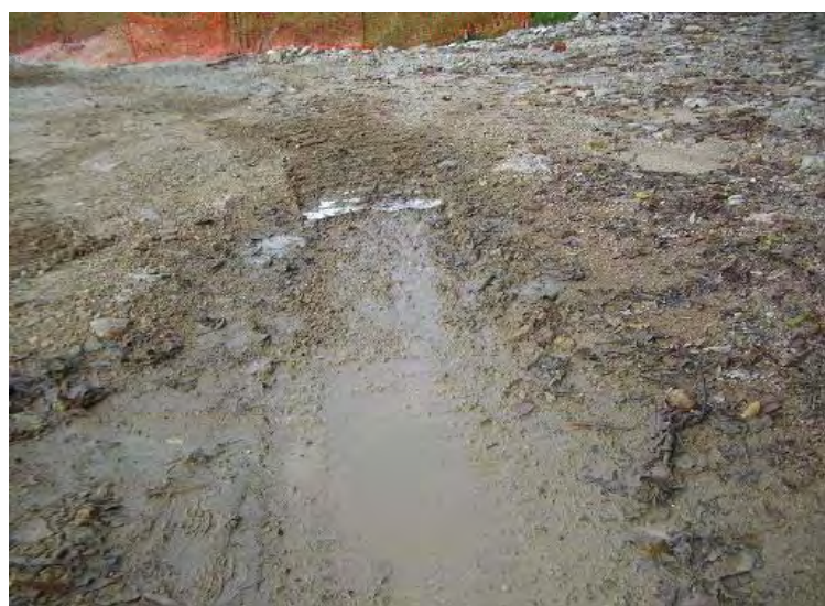
Stagnant water has been removed at MUP01/02.
