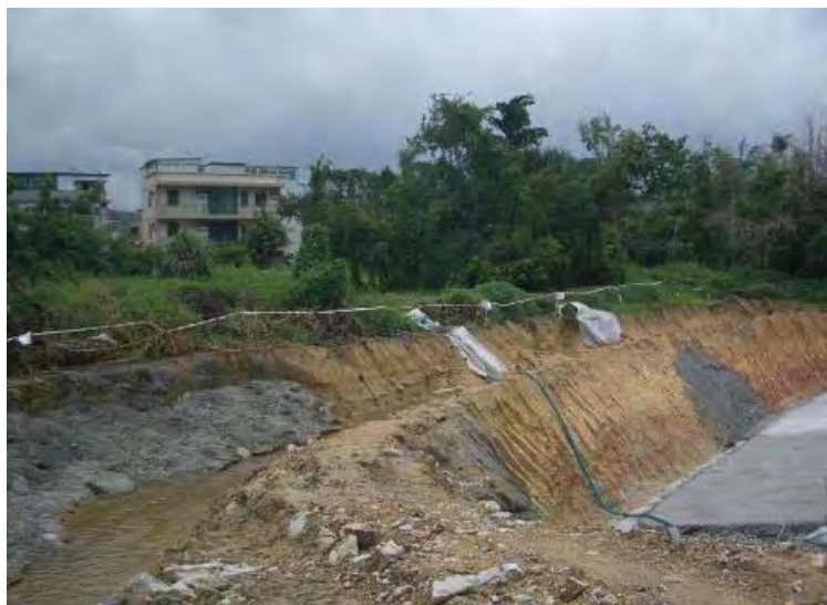
Damaged earthbound has been rectified at TKL02.
