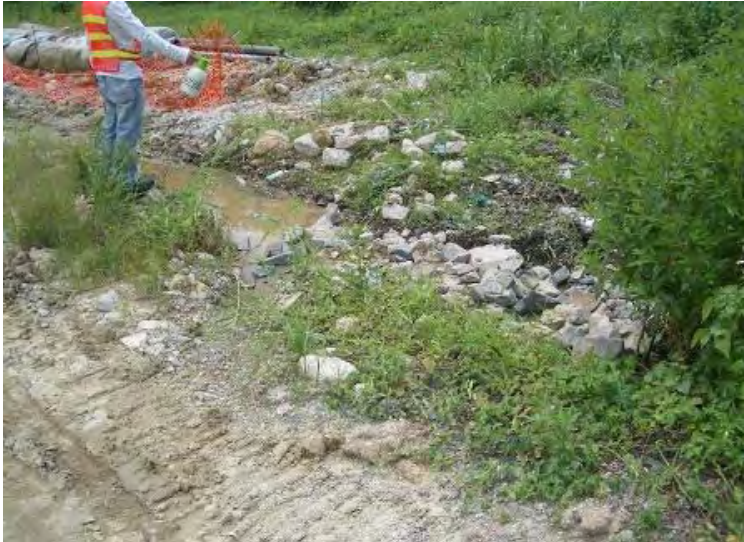
Stagnant water was removed at TKL07.
