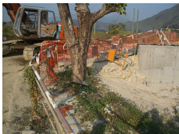
Exposed chemical containers were removed at TKL07.
