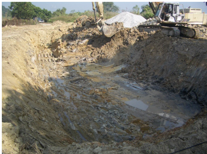
Stagnant water Stagnant water at TKL02 was cleared.
