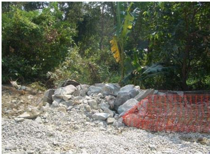
Stagnant water was cleared at MUP01/02.
