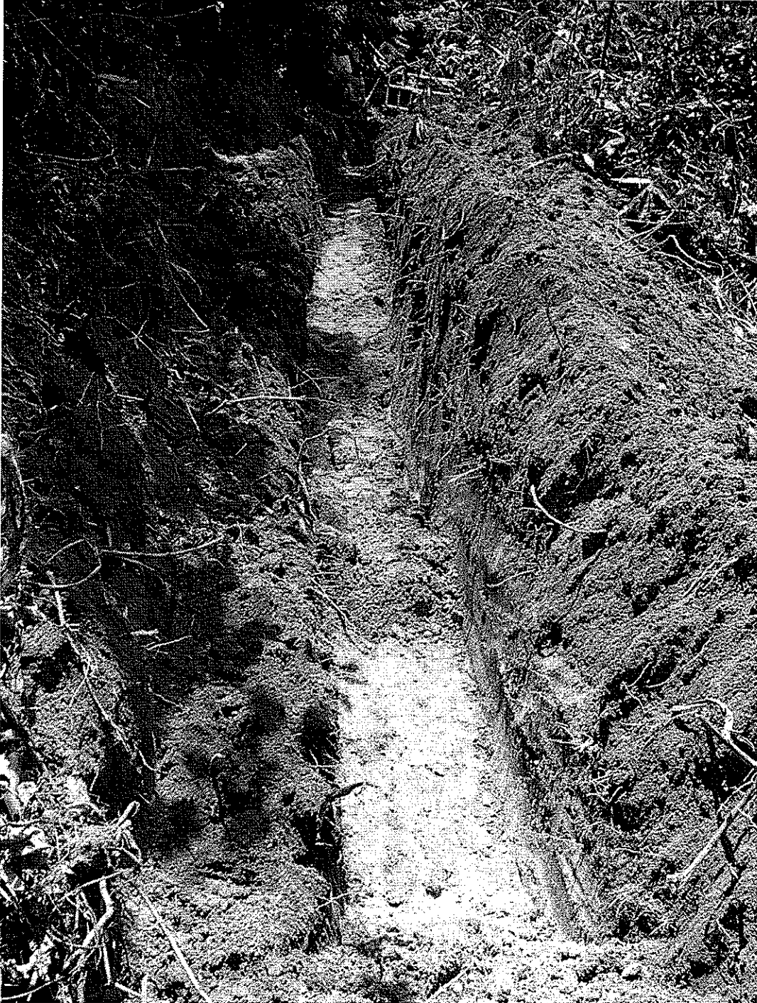
Plate 1: Overview of the machined alignment looking from MH S54 uphill towards MH S52 in the distance
