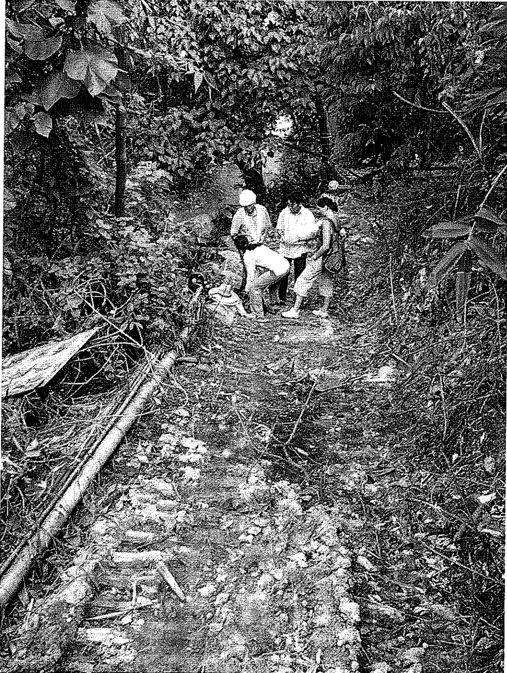
Plate 1: Pre-excavation view of the alignment between MHs S52 and S54 – looking north
