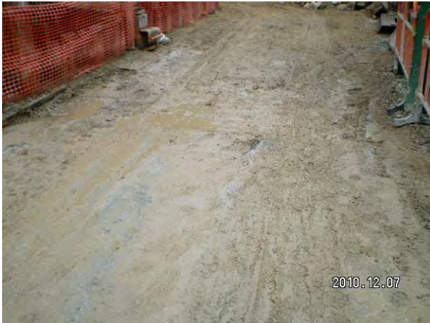
The Contractor should remove the mud and runoff water to keep the site access clear.
