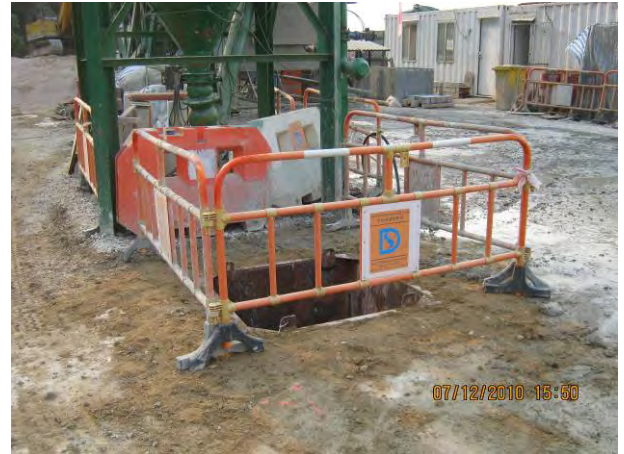
The well was built to direct and receive runoff water as to prevent further runoff to the access.
