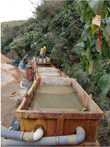
The filter sheets in the sedimentation tank should be kept cleaning regularly to maintain their function.
