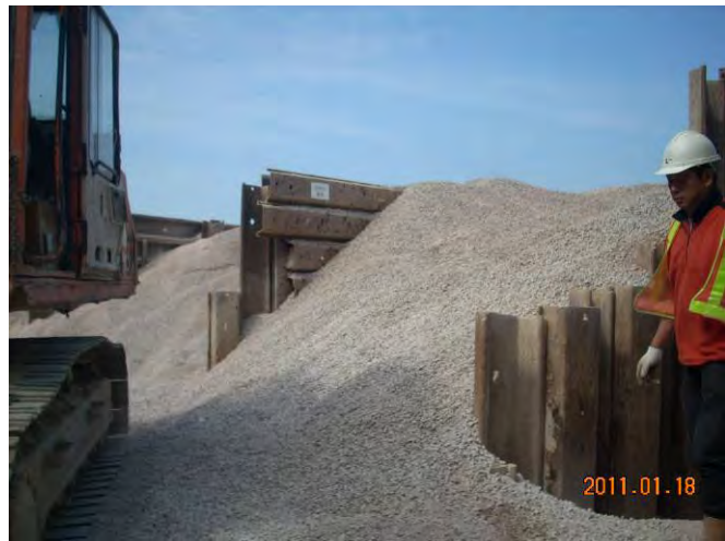
Water sprinkling should be applied on the concrete plant material to minimize dust nuisance.
