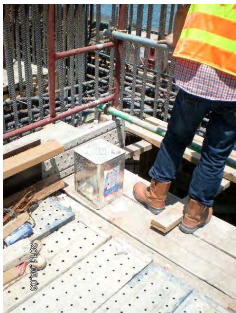
The Contractor should place the oil container to proper storage area after use.
