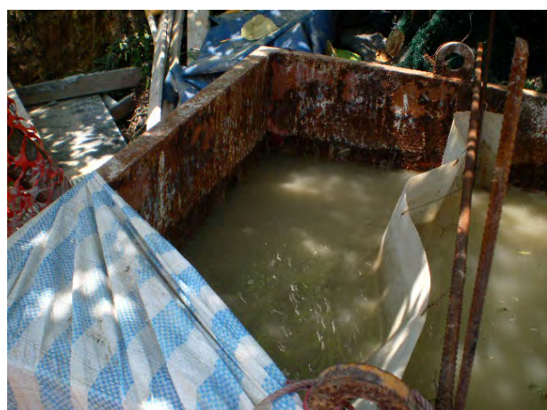
The sedimentation facilities need to be further modified to improve the de-silting effectiveness.
