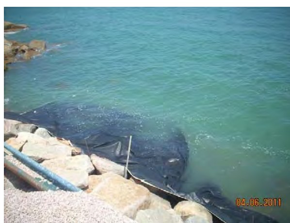
More silt curtains were observed setting up along the sea bank and no turbid water was observed. (Rectified on 4-6-2011)
