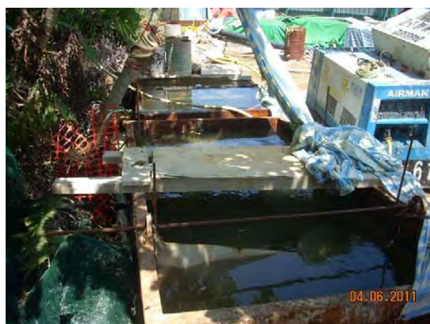
The water quality in the sed-tank was improved. (Rectified on 4-6-2011)
