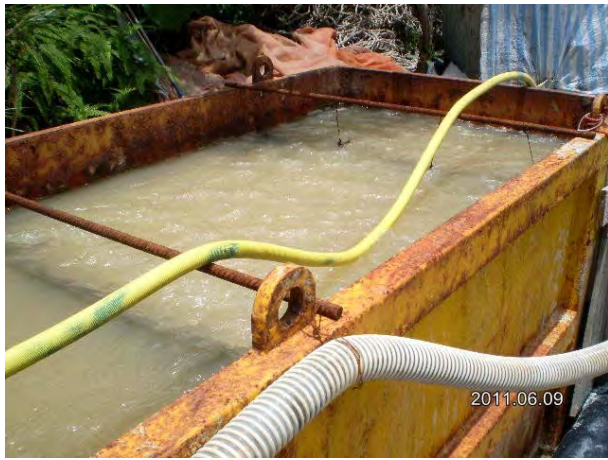
Overflow of turbid water was observed. The sedimentation facilities need to be further modified to improve the de-silting effectiveness.
