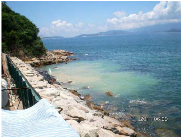
Turbid water was observed at the outfall of the site. The Contractor should carry out immediate action to rectify the problem of water quality.
