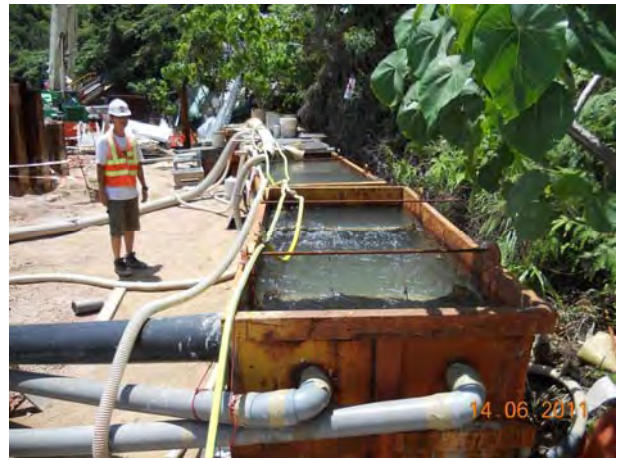
The water quality in the sed-tank was improved. (Rectified on 14-6-2011)
