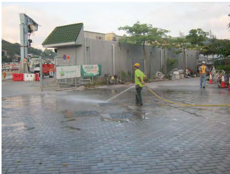
Photo B4: Photo record for mitigation measures provided by the Contractor at the site exit/entrance
