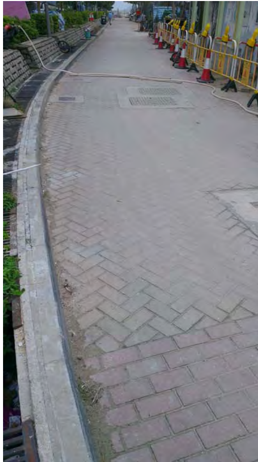
Photo B3: Photo record for dusty road outside ASD's work site
