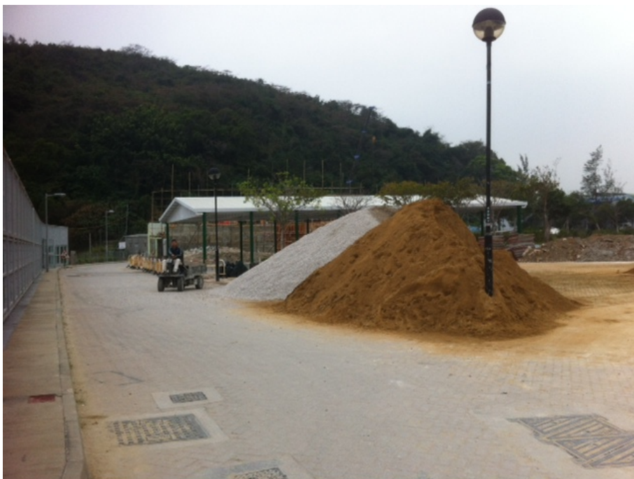
Photo B2: Photo record for sand and aggregate stockpiled next to the Yung Shue Wan playground and ASD's work site
