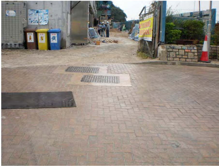
Photo B1: Photo record for air quality mitigation measures provided by the Contractor regularly
