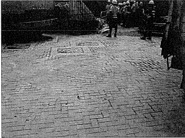
Photo 1 Dusty material was spread on the road at the entrance of the pumping station, the Contractor was reminded to wash the road regularly.
