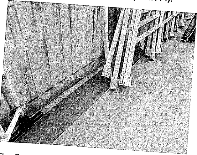
The Contractor was reminded to clean up the stagnant water at U-channel after rainy day.
