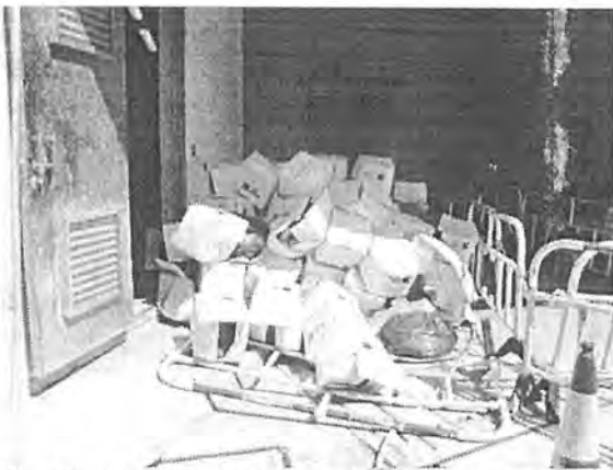
The Contractor was reminded to improve the housekeeping of the construction site.
