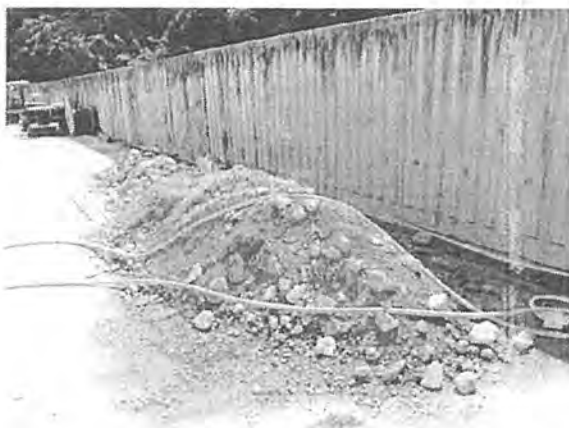
The Contractor was reminded to cover the stockpile with tarpaulin sheet to reduce dust generation.
