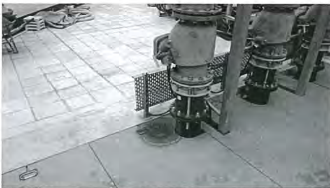
The Contractor was reminded to ensure no leaking of water from the junction of pipe at rooftop of YSW sewage treatment plant to avoid mosquito breeding.
