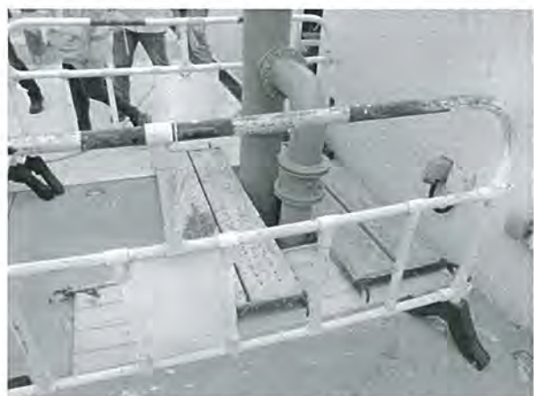
The opening of the water tank has been better covered.
