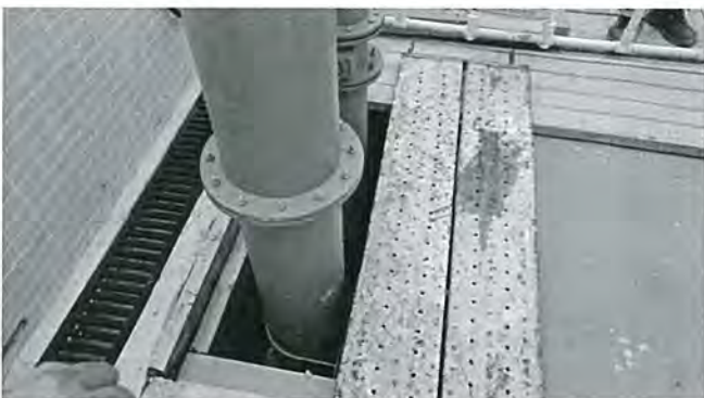
The Contractor was reminded to better cover the opening of water tank to prevent stagnant water being stored.
