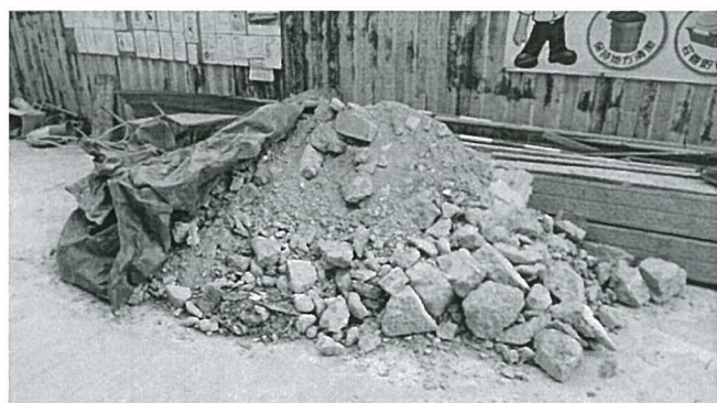
The Contractor was reminded to cover the stockpile well to reduce dust generation.
