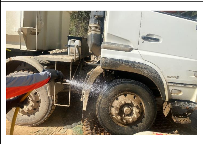
Wheel washing facilities with high pressure water jet provided at Site Entrance/Exit of Portion A
