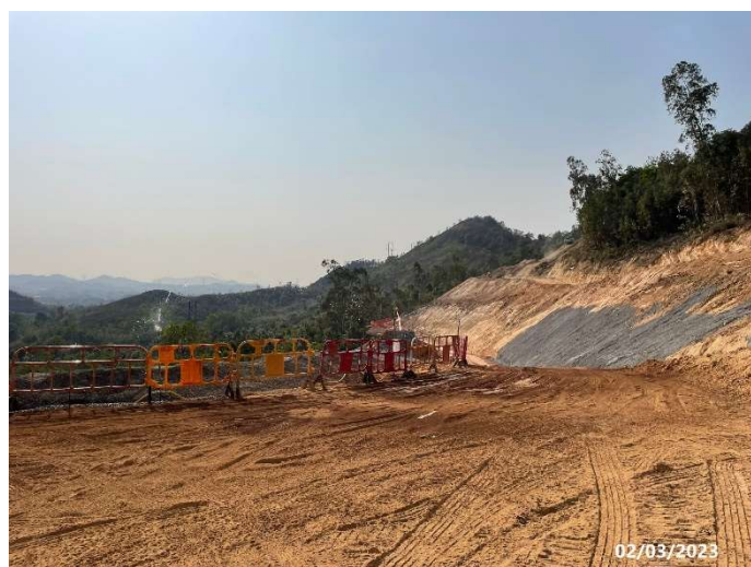
Photo 5 Water spraying by sprinklers at Portion A
