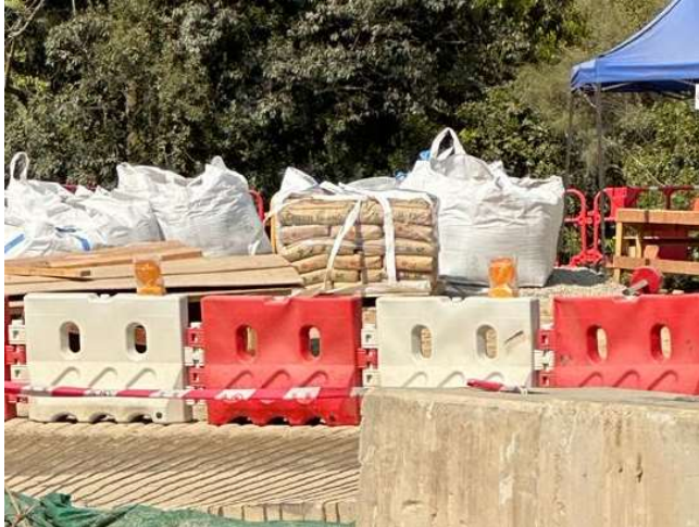
3. More than 20 bags of cement were not covered entirely by impervious sheets in SBA.
