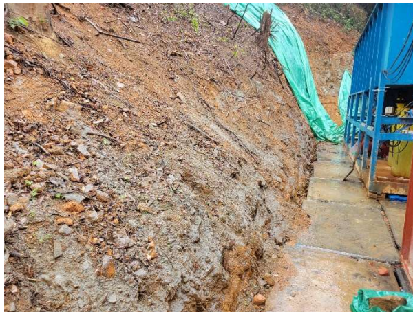
The chemical containers were removed. The Contractor has been reminded to store chemical containers properly.
