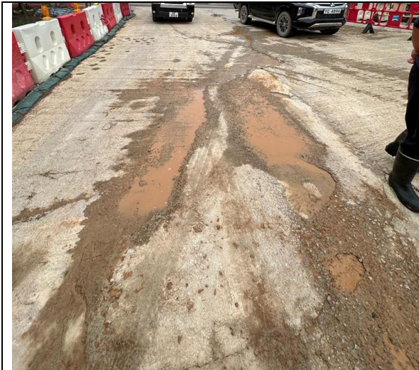
3. The entrance of Portion A is observed muddy.
