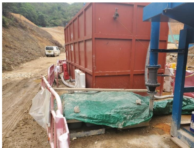
The chemical containers were placed in the drip and covered with impervious sheets.
