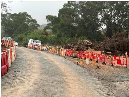
2. Sand and silt are observed at the vehicle entrance in SBA.
