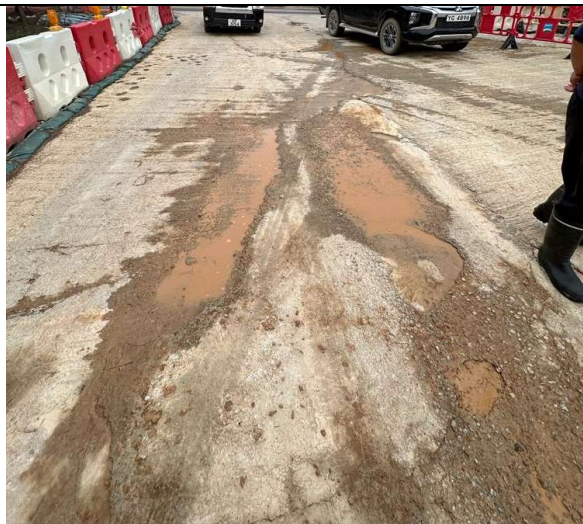
4. The entrance of Portion A was observed muddy.
