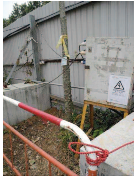
Photo 6 - A mobile distribution board was found inside TPZ.
