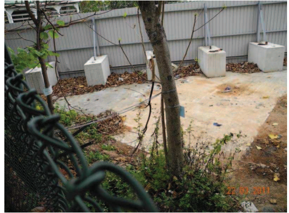
Photo 2 - A line of hoardings has also been erected in the western part of Area B, falling within the northwestern part of the Nursery.
