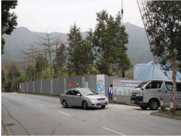
Photo 1 – Construction hoardings have been erected in Area A along the entire site boundary.
