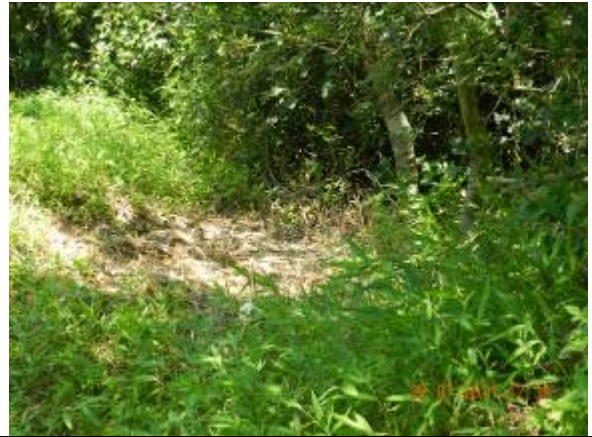
Photo 2 - The Contractor was informed and removal of such drainage pipe was observed
