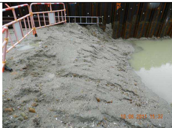
Photo 1 – Subsoil from area in Contract 2 was inspected by the Wetland Specialist on 10th August 2011.
