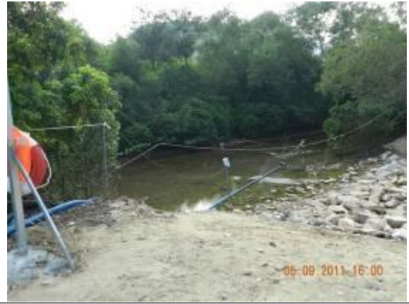
Photo 2 – The Pond of the Ecological Compensatory Area was observed to be connected to Wai Ha River directly.
