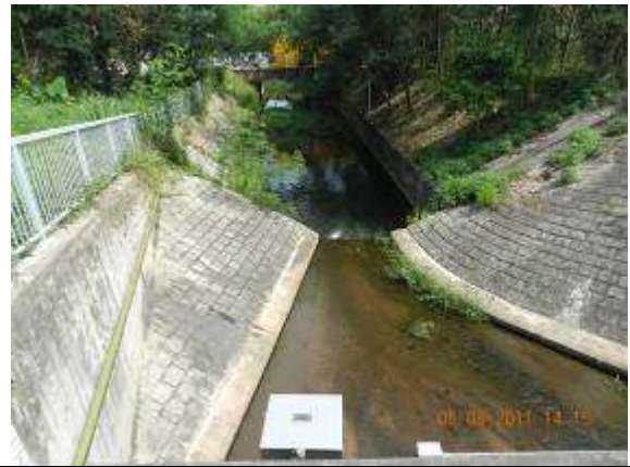
Photo 4 – Upper stream of Wa Ha River. No direct water discharge into the Wai Ha River since no active works area has been set up adjacent to the River.
