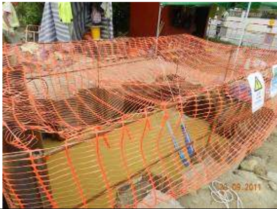
Photo 3 – Sedimentation tank for drained water from underground
