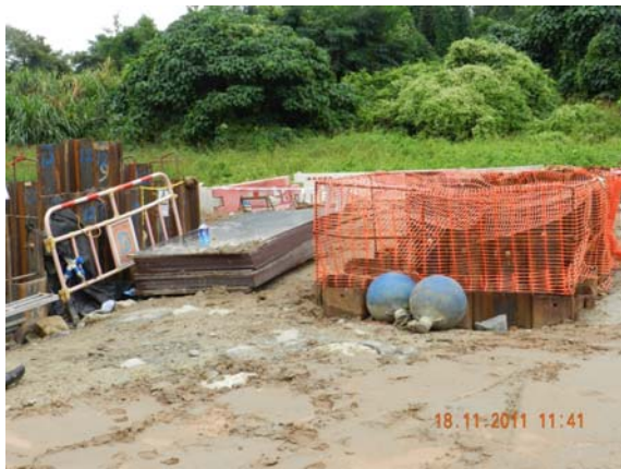
Photo 3 – Sedimentation tank for water drained from the underground
