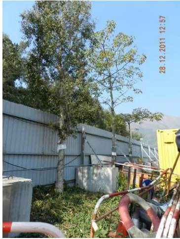
Photo 5 – Large construction materials that were temporarily stored within the TPZs were removed in Area A.
