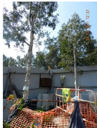
Photo 4 – Large construction materials that were temporarily stored within the TPZs were removed in Area A.
