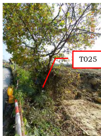
Photo 10 – No proper TPZ has been established around the Tree T025 and stockpiled soil was observed around the tree trunk base.
