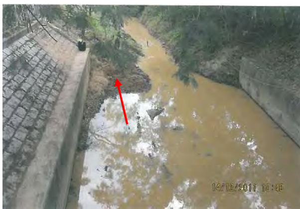
Photo 7 – Soil was stockpiled at the bank of the Wai Ha River for the excavation work (Photo provided by the Main Contractor).
