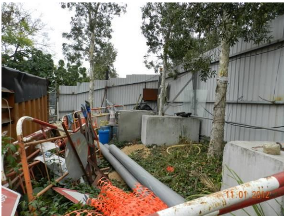
Photo 7 – Temporary stored construction materials were observed within the TPZs.
