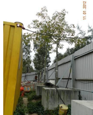
Photo 6 – Temporary stored construction materials were observed within the TPZs in Area A.
