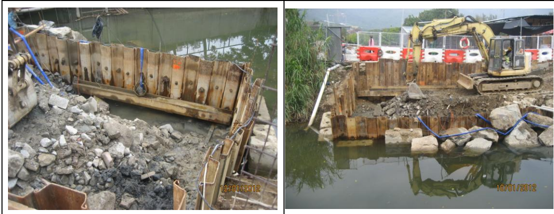
Photo7. The barrier was installed to avoid site water release to the river
