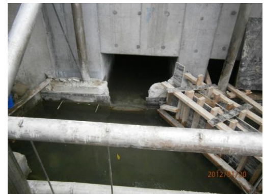
Photo6. River was redirect and narrowed causing high speed of water current.
