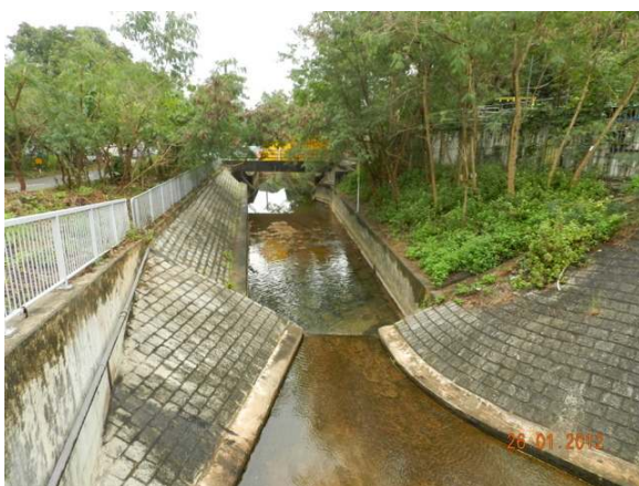
Photo 5 – Upper stream of Wa Ha River. No direct water discharge into the Wai Ha River since no active construction work from the Project has been commenced adjacent to the River.
