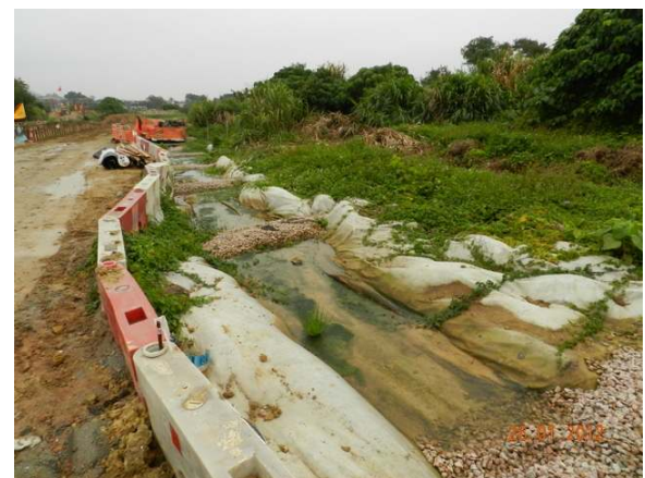
Photo 4 – Sedimentation tank for water drained from the underground.
