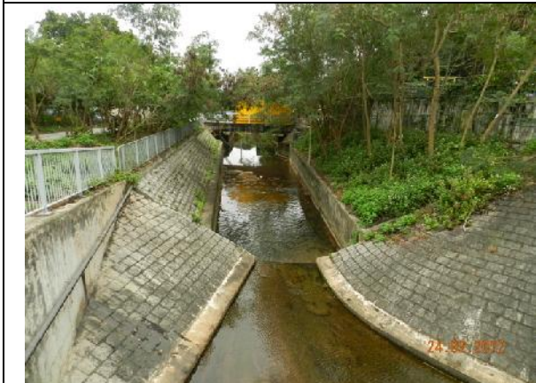
Photo 5 – Upper stream of Wa Ha River. No direct water discharge into the Wai Ha River since no active construction work from the Project has been commenced adjacent to the River.
