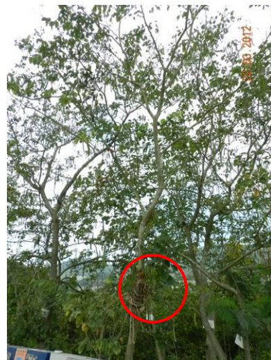
Photo 16 – The trunk of the retained tree U15 was found to be mechanically injured.
