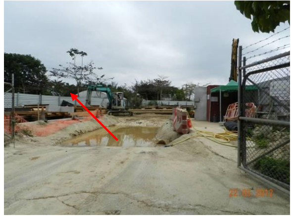
Photo 2 – A temporary hoarding was established to surround Area B within Tung Tsz Nusery.
