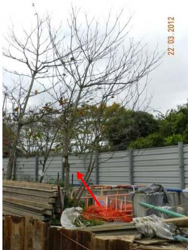
Photo 11 – Declining health condition of U34 in Area B.
