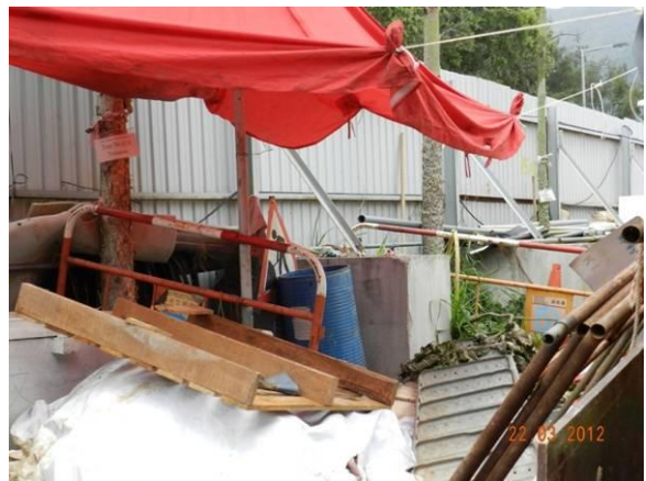
Photo 6 – Temporary stored construction materials were observed within the TPZs in Area A.
