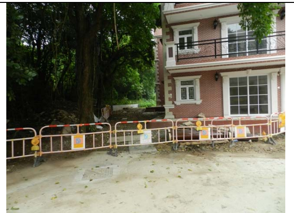
Photo 4 – Temporary hoardings were found erected at the northwest of the Treasure Spot Garden II on 19 th April 2012.
