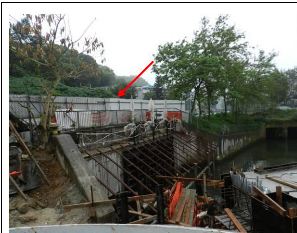
Photo 1 – A temporary hoarding was established to surround the work at Wai Ha River estuary.
