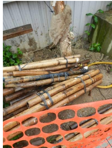
Photo 10 – Stockpiling of construction materials were observed close to the trunk of E22 within the TPZ.
