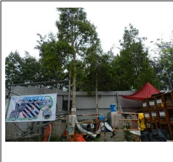
Photo 7 – Temporarily stored construction materials were observed within the TPZs in Area A.
