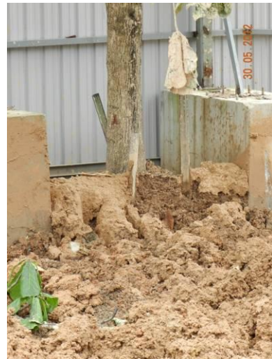
Photo 18 – Excessive soil was piled at the trunk base of a Terminalia catappa without tree tag.
