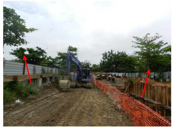
Photo 2 – A temporary hoarding was established to surround Area B within Tung Tsz Nursery.
