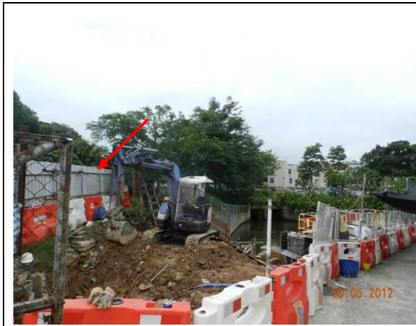
Photo 1 – A temporary hoarding was established to surround the works area at Wai Ha River estuary.
