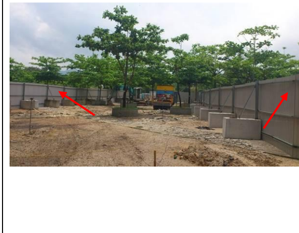
Photo 3 – A new section of temporary hoarding has been erected from southwest to eastern parts of the Tung Tsz Nursery.
