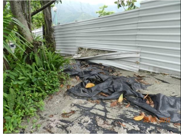
Photo 26 – Piled soil inside the works area was found spreading towards U50 through the broken site hoarding
