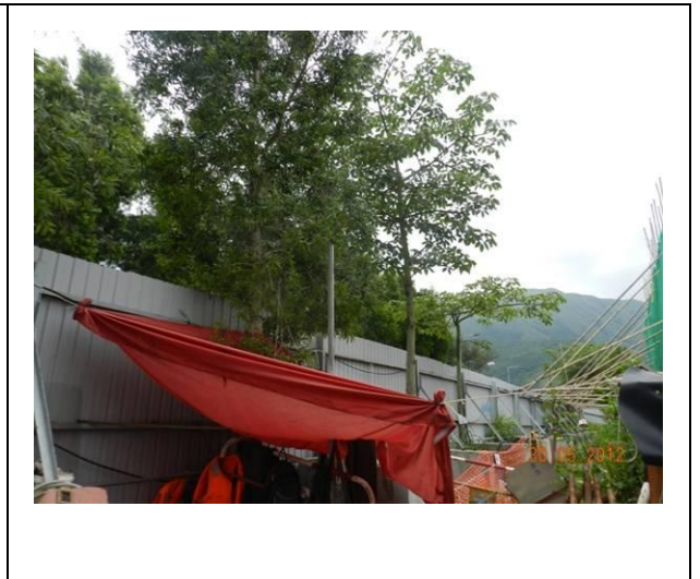
Photo 8 – Temporarily stored construction materials were still observed within the TPZs in Area A.
