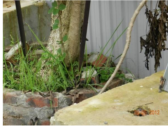
Photo 20 – The planter of U70 was found partially broken for the establishment of the temporary site hoarding.
