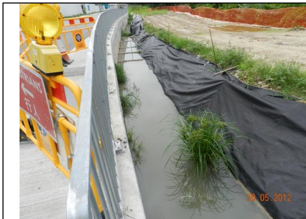
Photo 7 – The sedimentation beds and PVC liner were aligned from western to eastern parts along Tung Tsz Road and opposite to San Tau Kwok.
