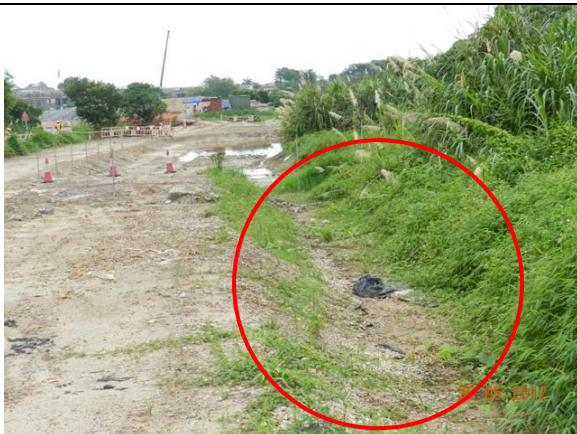
Photo 5 – The sedimentation beds aligned along the boundary of the works area to the south of Wai Ha was removed.
