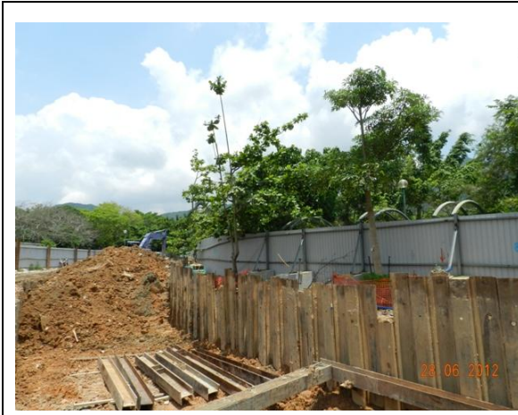
Photo 19 – Relocated trees were unable to be assessed closely due to the construction of the box culvert.
