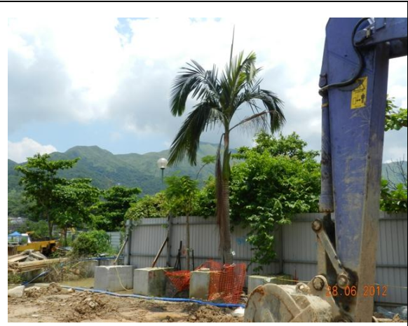
Photo 26 – The guying ropes of A36 were removed and the palm was slightly leaning.
