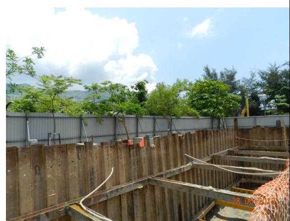
Photo 18 – Relocated trees were unable to be assessed closely due to the construction of the box culvert.
