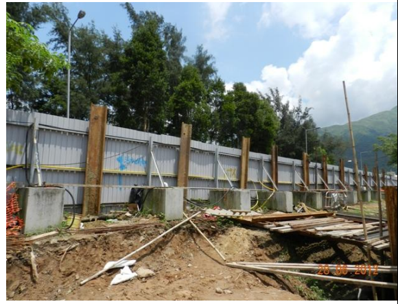
Photo 8 – Sheet piling work was observed within the TPZs at the southwestern part of Area A.
