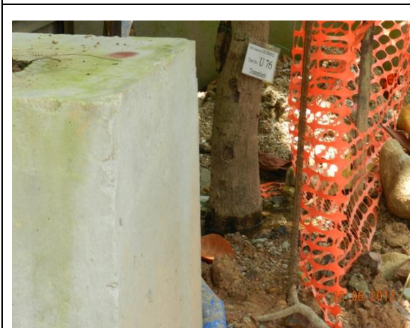
Photo 23 – Waterlogged area was observed at the base of U76.
