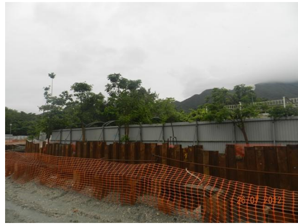
Photo 16 – Relocated trees were unable to be assessed closely due to the construction of the box culvert.
