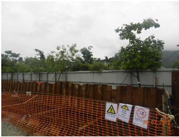
Photo 15 – Relocated trees were unable to be assessed closely due to the construction of the box culvert.
