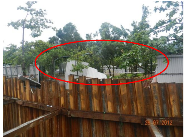
Photo 4 – Site hoarding was found collapsed in Area B.
