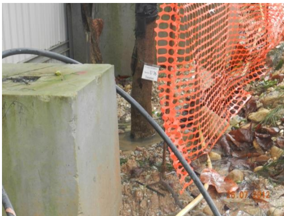
Photo 17 – Waterlogged area was observed at the base of U76.
