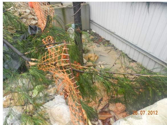
Photo 18 – Waterlogged area was observed at the base of U77.
