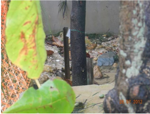
Photo 19 – Waterlogged area was observed at the base of U78.
