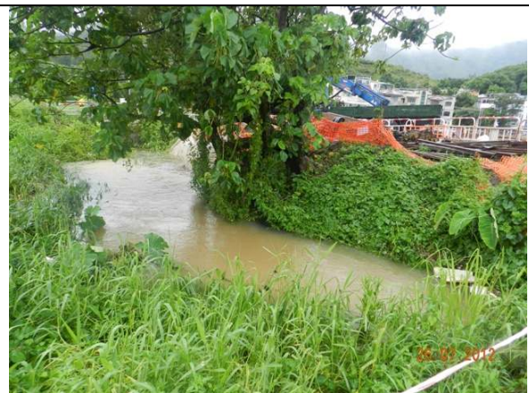
Photo 8 – The sedimentation beds and PVC liner were aligned from north to south near the retained tree T196 ( Macaranga tanarius var. tomentosa ).
