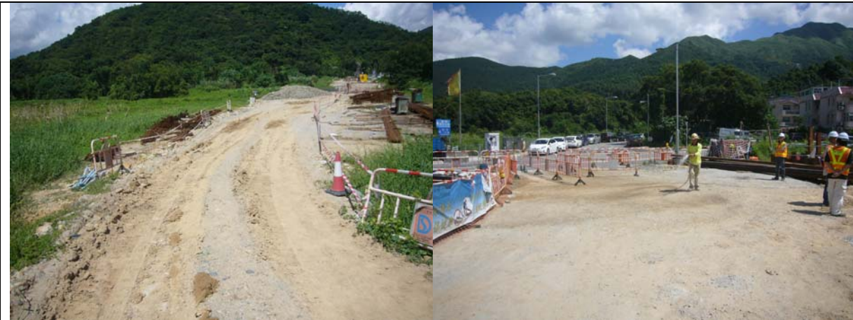
As a reminder, water spraying should be applied to the haul road and stock pile to minimize dust generation.
