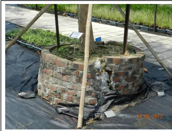
Photo 13 – Crack on the planter of U75 became more obvious in Area B.
