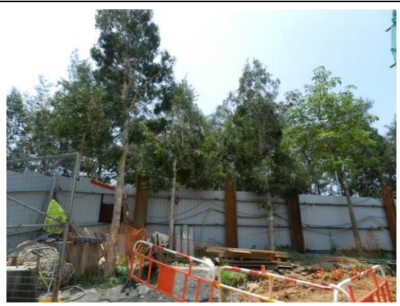
Photo 14 – No temporary storage of construction materials were observed within the TPZs in Area A.
