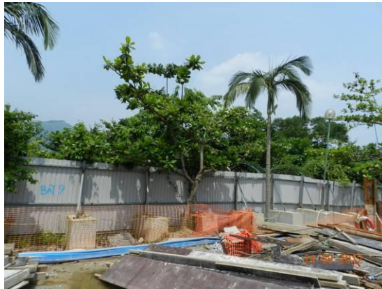
Photo 21 – General view of the relocated trees behind the sheet piles in Area B.
