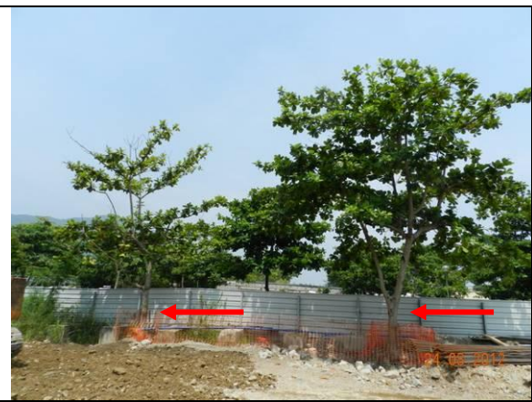
1.1.2 Photo 26 – U54 (left) and an untagged tree (right) have been surrounded by the orange construction nets to prevent further damage to the tree trunks.
