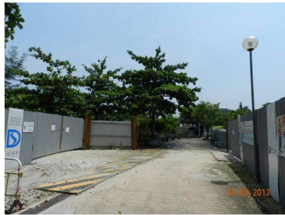
Photo 3 – Temporary hoardings has been erected to surround the new section of construction areas within the Nursery, an access road has been maintained for daily operation of the Nursery.
