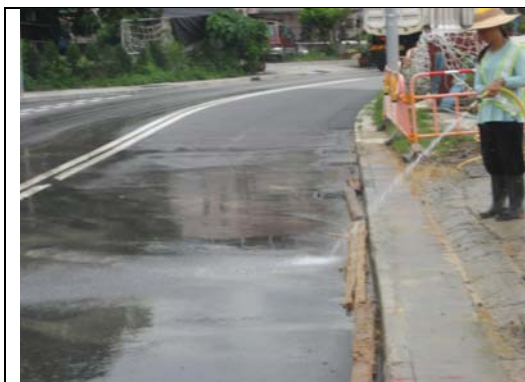
(Photo 1) Cleaning of site exit is observed and no wastewater from the wheel washing facility was found to be overflowed from site.
