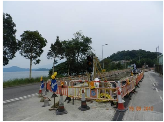
Photo 2 – Temporary hoardings have been established to active works area along Ting Kok Road.
