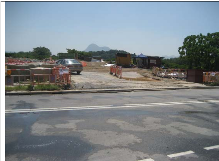
1. Water spraying was observed at the site exit/ entrance.
