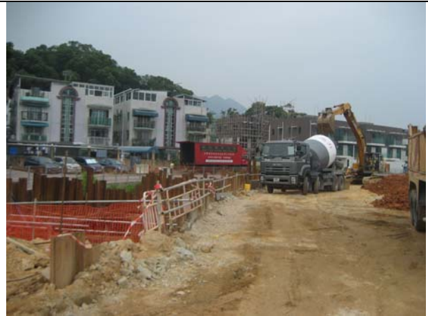
2. Watering was found to be applied on the dry haul road.
