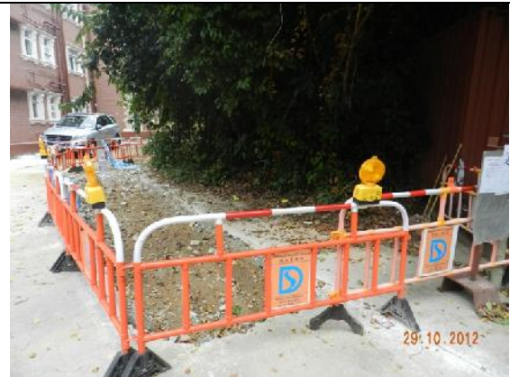
Photo 4 – New temporary hoardings have been erected on the path outside Treasure Spot Garden II.
