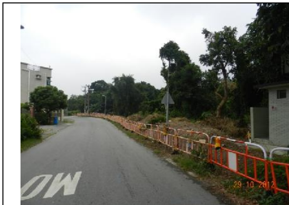
Photo 1 – Temporary hoardings have been erected around the active works area to the south of Wai Ha.
