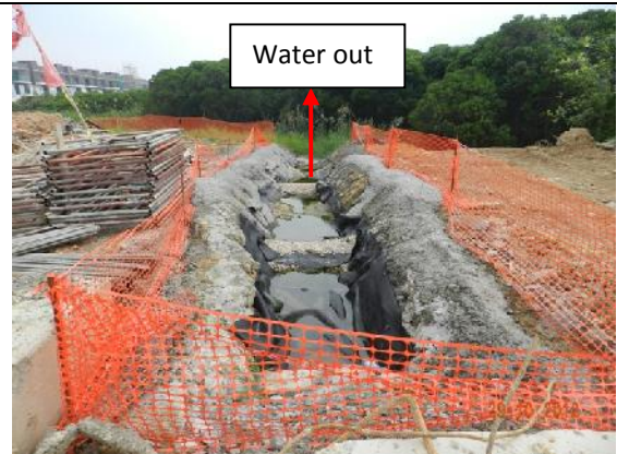
Photo 10 – New section of sedimentation beds with gravels and PVC liners was found aligning from the area opposite to the Jade View Villa towards the marsh area at southeast.
