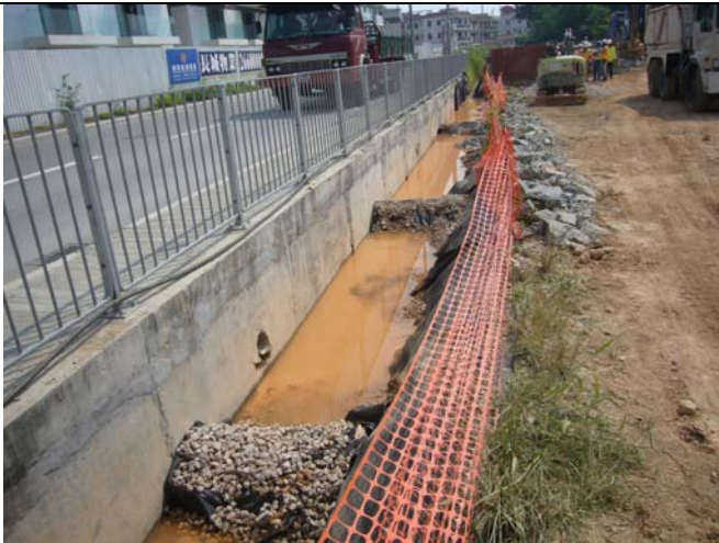
Photo 3: The sediment inside the de-silting channel should be cleared regularly in order to maintain its function.
