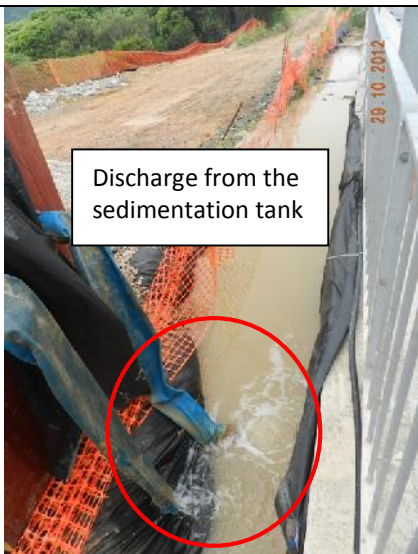
Photo 11 – Muddy water drained from the excavated site opposite to San Tau Kok.
