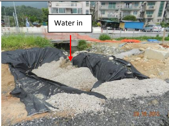
Photo 9 – New section of sedimentation beds with gravels and PVC liners was found aligning from the area opposite to the Jade View Villa towards the marsh area at southeast.
