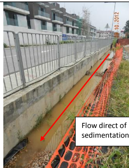
Photo 12 – Muddy water drained from the excavated site opposite to San Tau Kok.
