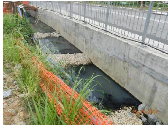
Photo 8 – The sedimentation beds and PVC liner were aligned from western to eastern parts along Tung Tsz Road and opposite to San Tau Kwok and no muddy water was discharged.
