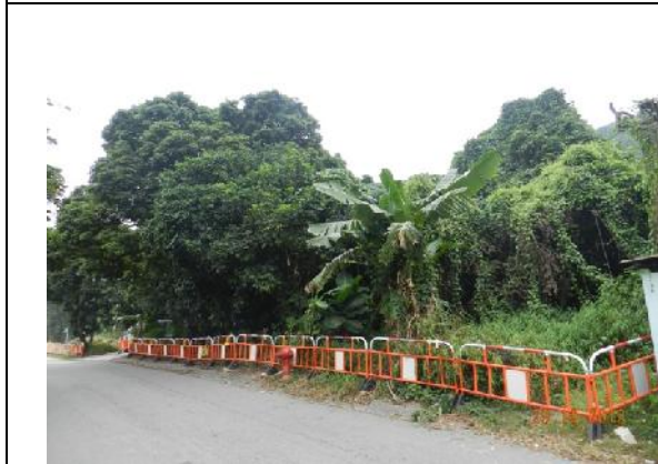
Photo 3 – New temporary hoardings have been erected along the west of Tung Tsz Road near the refuse collection point.
