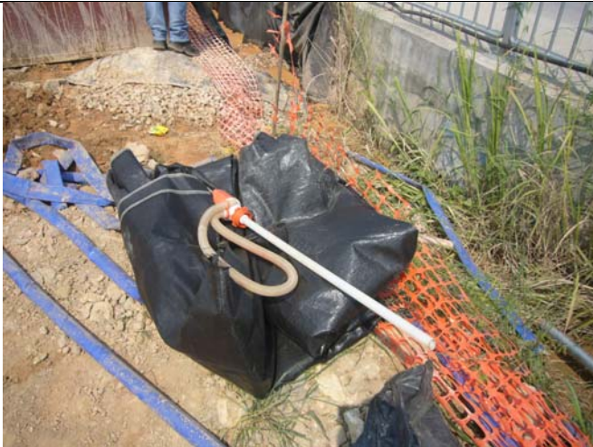
Photo 4: Chemical waste was observed on bare ground, the Contractor should store the chemical waste in proper area before dispose of.
