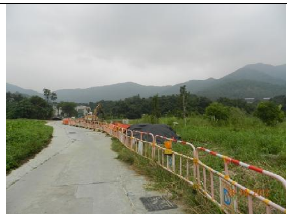
Photo 2 – Temporary hoardings have been erected around the active works area along access road to Treasure Spot Garden II.
