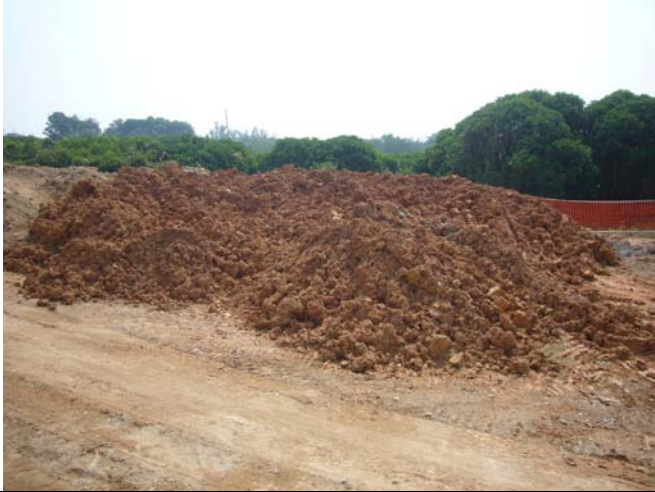
Photo 2: Opened stockpile was observed, the Contractor should provide impermeable cover on it to minimize dust impact.
