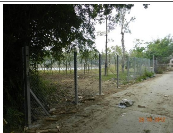
Photo 2 – A new set of chain link fence has been erected at the previous entrance of Area C after the handover to AFCD.
