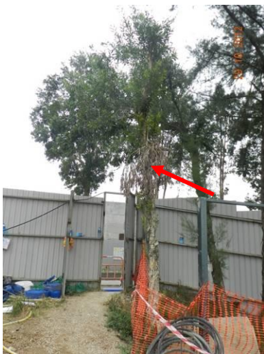
Photo 11 – A broken scaffold branch was observed on the tree to be transplanted (T102) in Area B.
