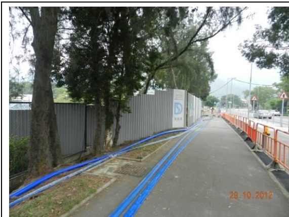
Photo 1 – Temporary hoardings have been established along Ting Kok Road outside Tung Tsz Nursery.
