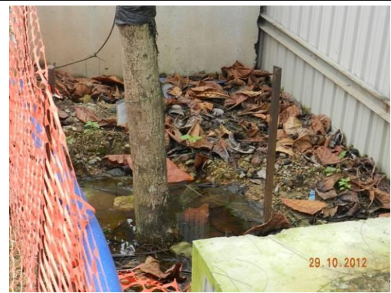
Photo 16 – Waterlogged area was observed at the base of the relocated tree U6 in Area B.
