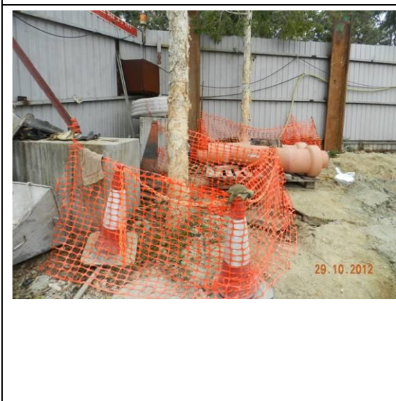
Photo 5 – No temporary storage of construction materials were observed within the TPZs in Area A.
