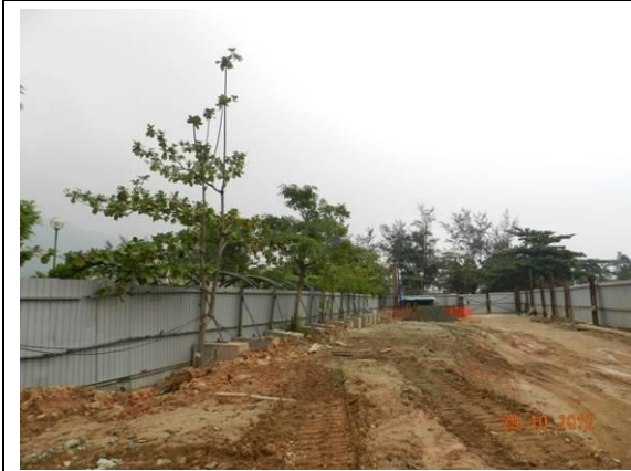
Photo 15 – No proper tree protection zones were set up along the transplanted tree in Area B.
