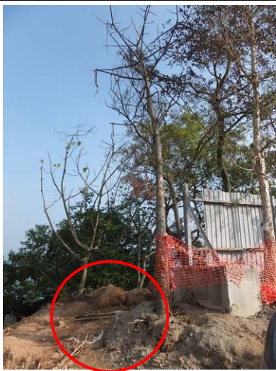
1.1.1 1.1.2 Photo 8 – Excavation works near the relocated E17 and exposed the roots of the tree were found.
