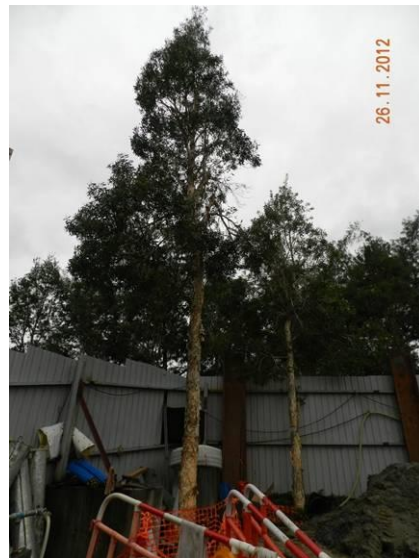
Photo 6 – No temporary storage of construction materials were observed within the TPZs in Area A.
