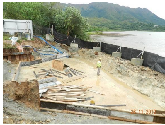
Photo 1 – Temporary hoarding of the northeastern part of Area A was extended outward.
