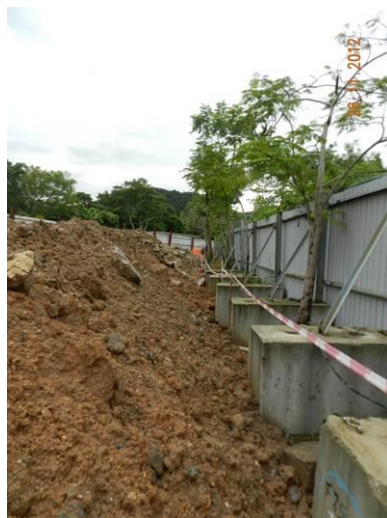
Photo 18 – No proper tree protection zones were set up along the transplanted trees in Area B.
