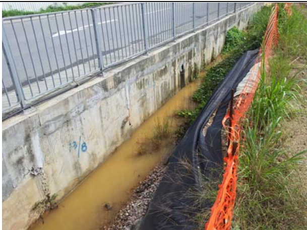
Photo 1 : The sediment inside the de-silting channel should be cleared regularly in order to maintain its function.
