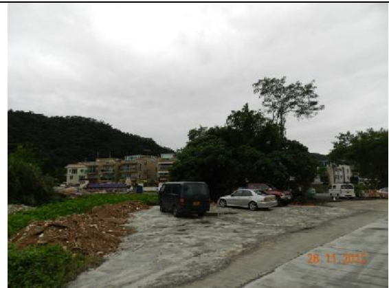
Photo 6 – A newly paved area was created for parking next to the retained tree groups (T088 – T091).
