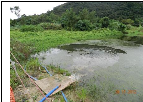
Photo 13 – Discharge of filtered water from the works area into the wetland rehabilitation area
