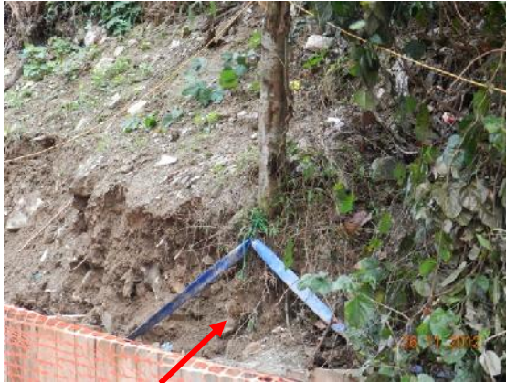
Photo 19 – Excavated work close to the retained tree T103 was observed and it covers almost half of the root zone area of the tree.
