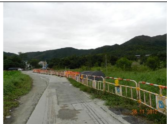
Photo 2 – Temporary hoardings have been erected around the active works area along the access road to Treasure Spot Garden II.
