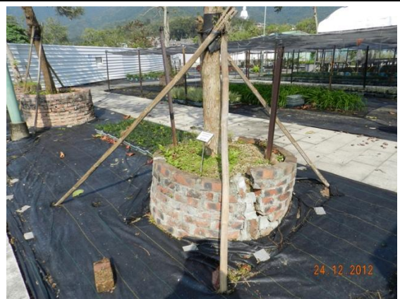
Photo 12 – Cracks on the planter of U75 became more obvious in Area B.
