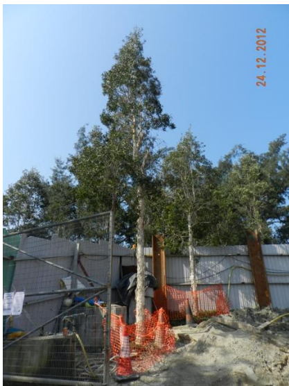
Photo 5 – No temporary storage of construction materials were observed within the TPZs in Area A.
