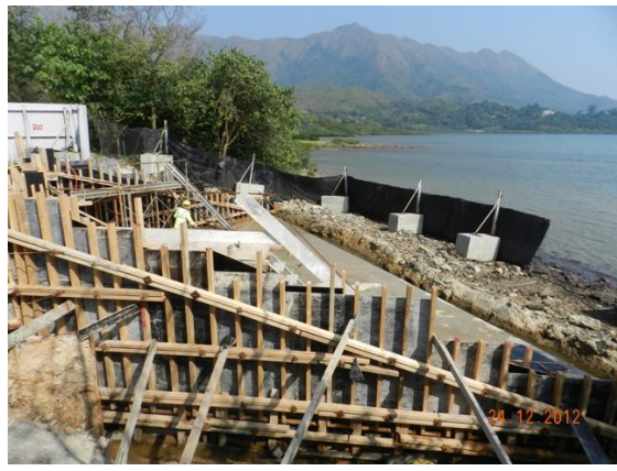
Photo 1 – Temporary hoarding of the northeastern part of Area A facing the sea.
