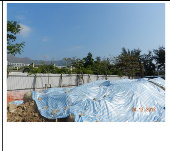
Photo 18 – Relocated trees were not inspected closely as piling of soil and stones were next to them.
