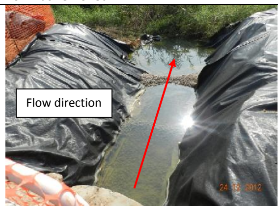
Photo 12 – The sedimentation beds with gravels and PVC liners was aligned from the area opposite to the eastern part of Jade View Villa towards the marsh area at southeast.
