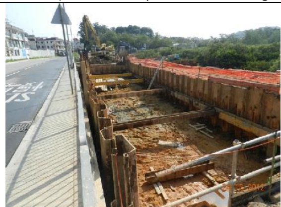
Photo 10 – The sedimentation beds and PVC liner originally aligned from western to eastern parts along Tung Tsz Road and opposite to San Tau Kwok was removed.
