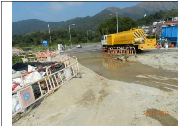
Photo 7 – Wheel washing facilities has been maintained at the vehicular exit point of the works area of Contract 2.
